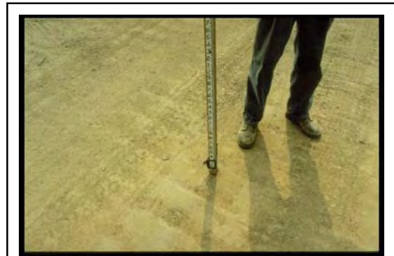
Fig. 3. Construction site with significant compaction of the deep basal till subsoil extends 24 inches below this exposed cut-and-fill work surface.
