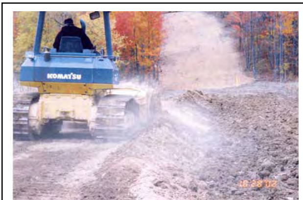
Fig. 12. Moderately dry topsoil is being replaced on the affected site now that Phase 1 deep ripping of the compressed subsoil is complete.
