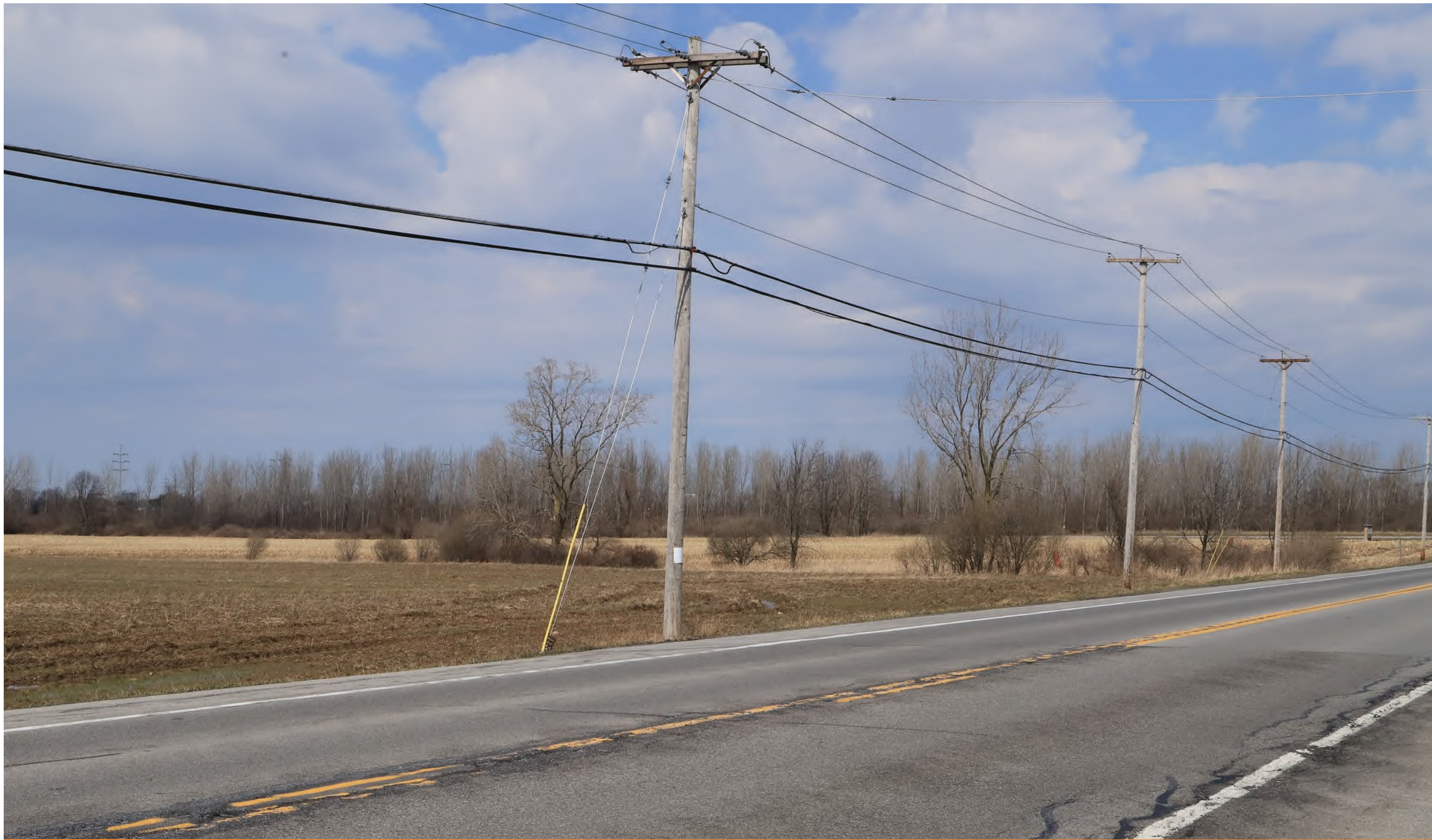
PHOTO 7 ALLEGHENY ROAD SIMULATED CONDITION
