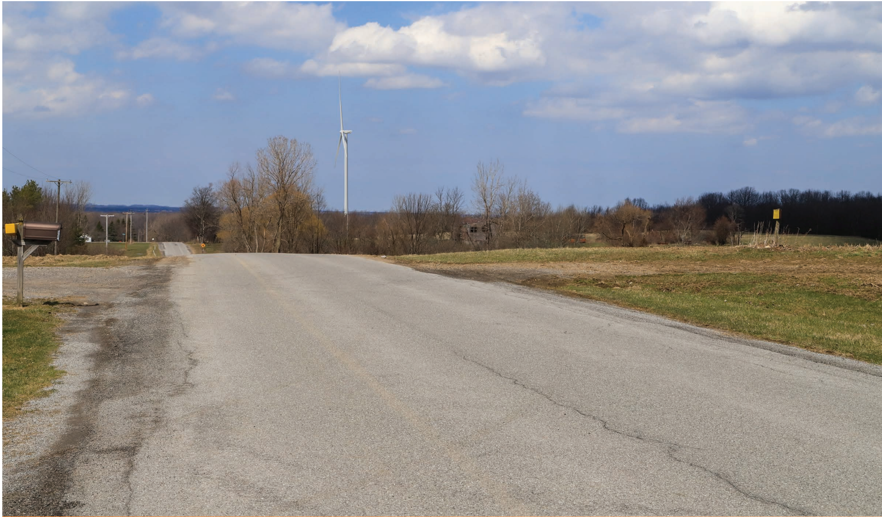
Photo 9 - Chaddock Rd near # 11080 SIMULATED CONDITION - 640
